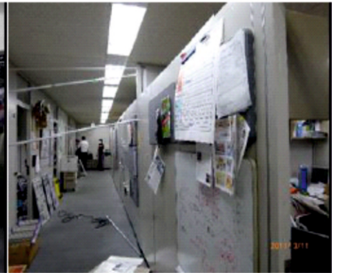
(c) Deformation of a partition wall
