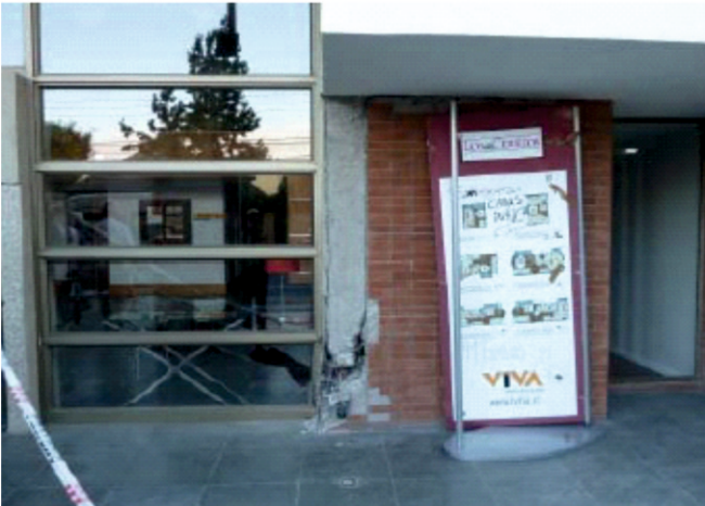
Photo4-2 Crushed column bottom
