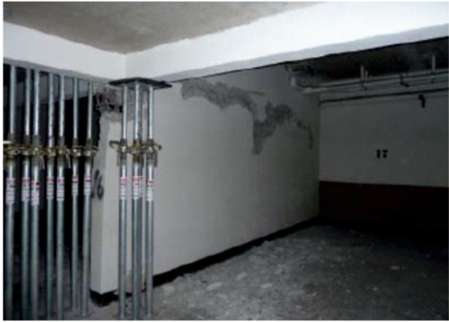
Photo 2-2 Smashed RC wall
