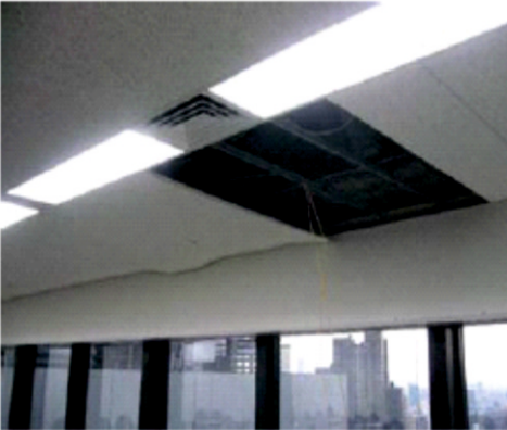
(a) Fall of ceiling panels
